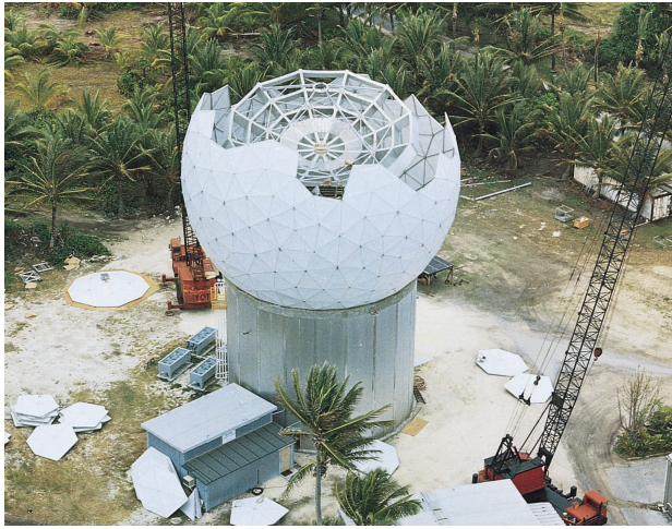
FIGURE 5. The forty-five-foot millimeter-wave (MMW) antenna and its sixty-eight-foot radome under construction on Roi-Namur Island at Kwajalein. The MMW radar was built to extend the general imaging and tracking capabilities of ALCOR and to develop millimeter-wavelength signatures of ballistic missile components.
