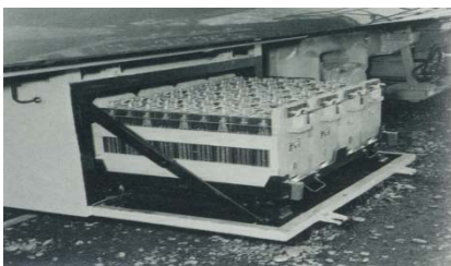
Fig 10 Ni-Cd batteries installed in electric trains of Kintetsu in 1958
