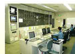
電力系統安定化技術 Electric Power System Stabilizing Technology
