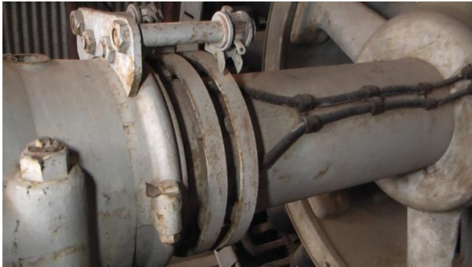
DC field slip ring (the field was on the rotor) wires carry DC power from the rings to the field coils
