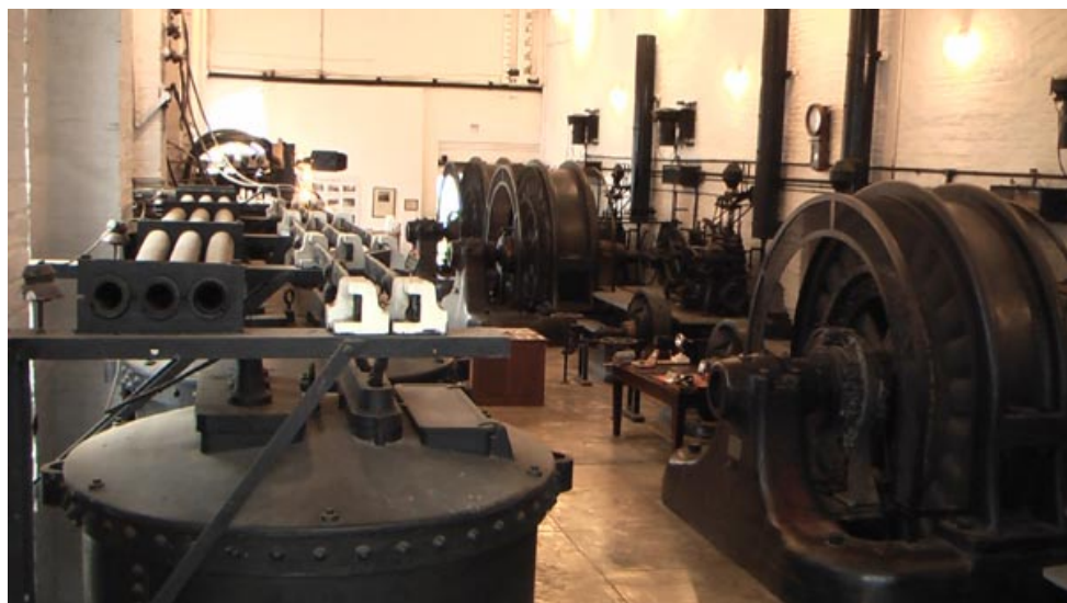
Wide view of the generator room
