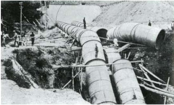
Fig. 2 Two penstock runs in the Keage Power Station.
